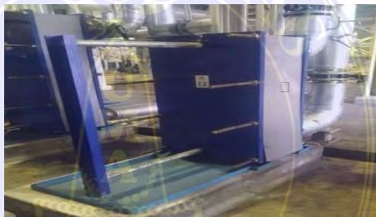
GAMBAR 3. 5 PLATE HEAT EXCHANGER
