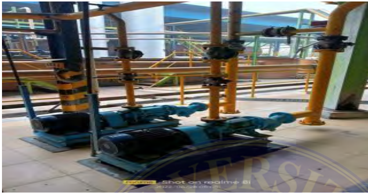
Gambar 3.6. Oil Pump final Transfer
