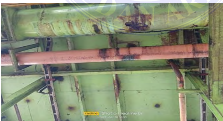
Gambar 3.30. Crude Oil Gutter
