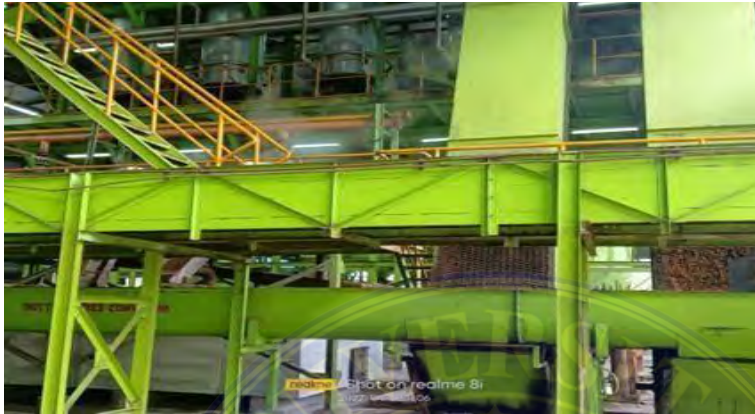
Gambar 3.29. Horizontal empty bunch conveyor
