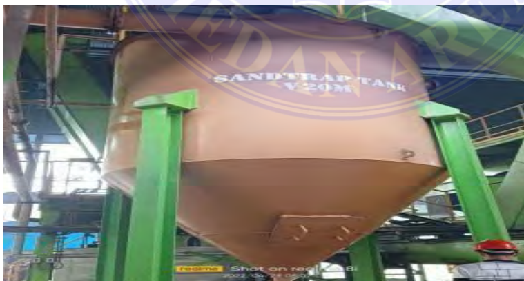
Gambar 3.5. Sand Trap Tank
