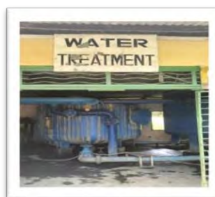
Gambar water treatment
