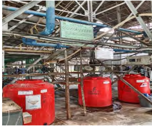
Gambar 3. 61 Pengolahan Air (water treatment)
