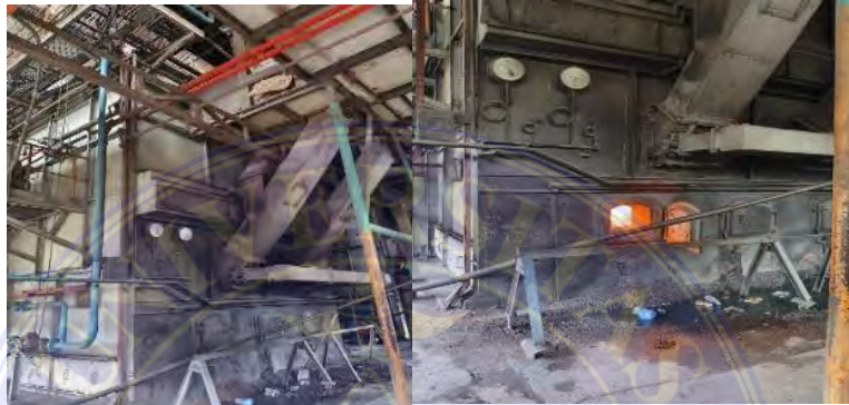
Gambar 3. 57 Ketel Uap (Boiler)
