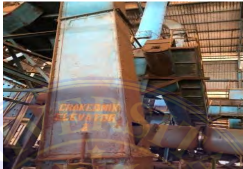
Gambar 3. 48 Cracked Mixture Elevator
