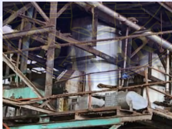
Gambar 3. 38 Continuous Settling Tank
