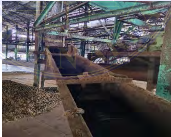
Gambar 3. 30 Inclide Distribusi Bunch Conveyor
