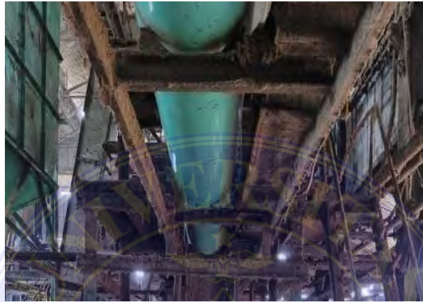
Gambar 3. 53 Under Silo Conveyor
