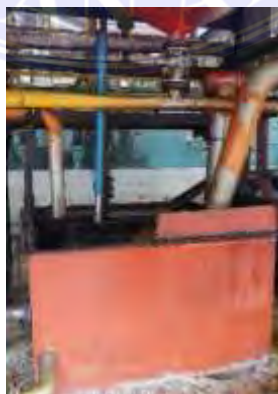
Gambar 3. 30 Sludge Drain Tank
