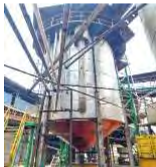
Gambar 3. 20 Vertical Clarifier Tank
