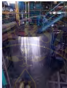
Gambar 3. 50 Feed Water Tank
