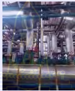
Gambar 3. 41 Back Pressure Vessel
