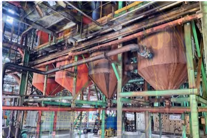
Gambar 3.37 Oil Purifier Tank
