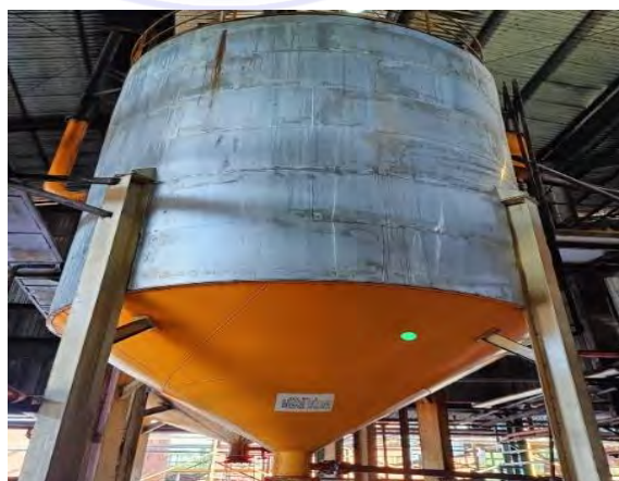
Gambar 3.36 Continuous Settling Tank (CST)
