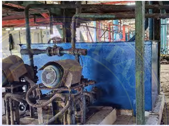
Gambar 3.46 Hot water tank
