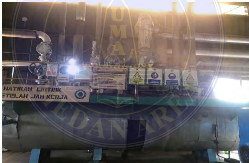
Gambar 3.45. Back Pressure Vessel
