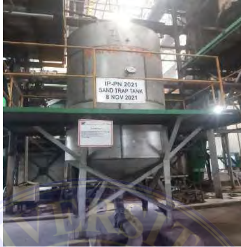
Gambar 3.25. Sand Trap Tank
