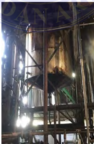
Gambar 3.27. Crude Oil Tank
