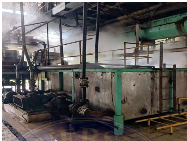
Gambar 3.12 Crude Oil Tank (Bak RO)
