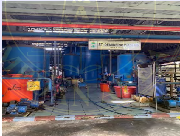
Gambar 3. 28 Water Treatment Plant
