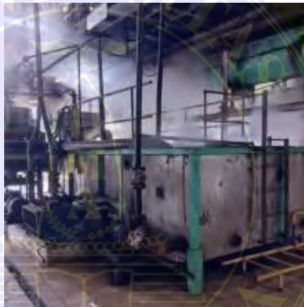
Gambar 3. 12 Crude Oil Tank (Bak RO)
