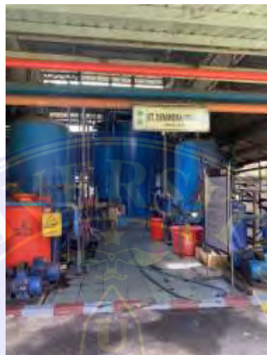
Gambar 3. 28 Water Treatment Plant
