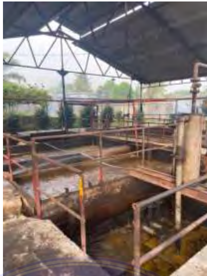
Gambar 3. 23 Bak Penampung Sludge ( Fat Pit )
