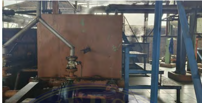
Gambar 3. 15 Light Phase Tank
