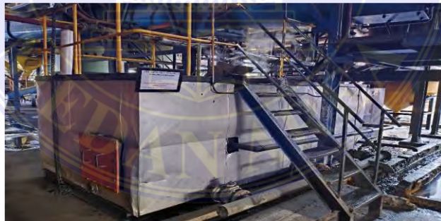
Gambar 3. 10 Crude Oil Tank
