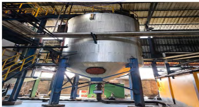
Gambar 3. 11 Continuous Settling Tank
