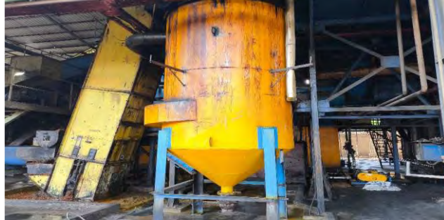
Gambar 3. 8 Sand Trap Tank
