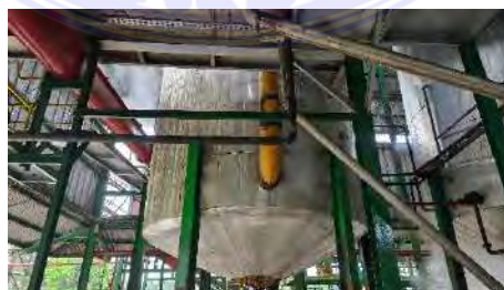
Gambar 3. 31. Continous Settling Tank
