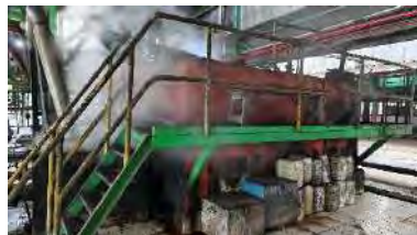
Gambar 3. 29. Crude Oil Tank
