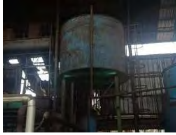
Gambar 3. 44. Boiler Feed Water Tank
