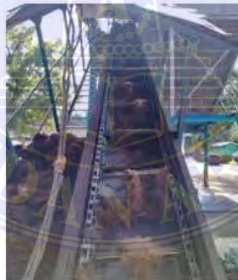
Gambar 3.12. Empty Bunch Conveyor
