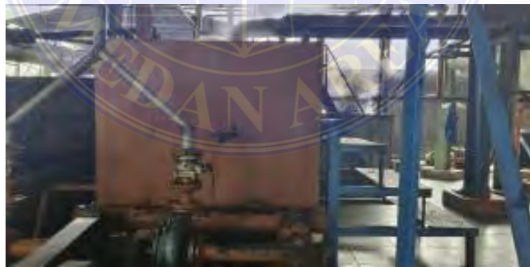
Gambar 3. 16 Light Phase Tank
