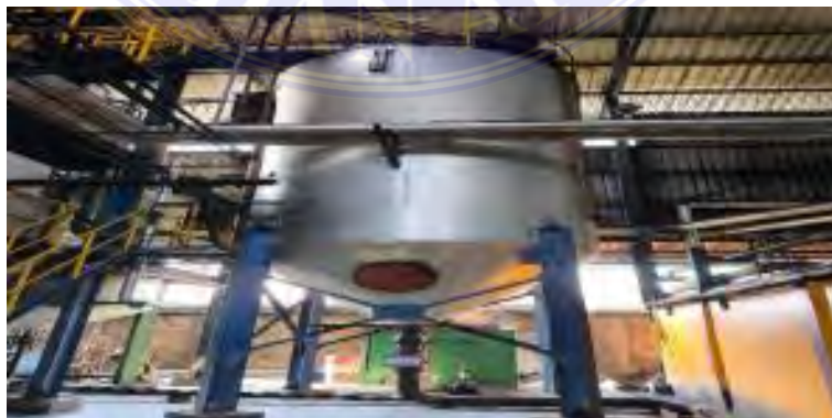
Gambar 3. 12 Continuous setting Tank
