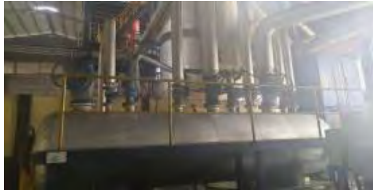
Gambar 3. 48 Back Pressure Vessel
