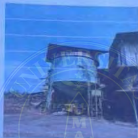
Gambar 3.31 Kernel Bulk Silo
