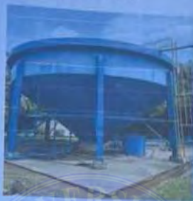
Gambar 3.33 Water Clarifier Tank
