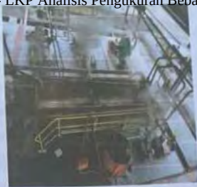
Gambar 3.21 Sludge Drain Tank
