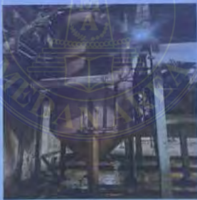
Gambar 3.12 Sand Trap Tank
