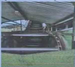
Gambar 3.4 FFB Scraper Conveyor
