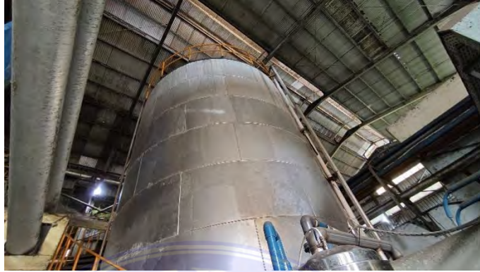
Gambar 3. 62 Feed Water Tank
