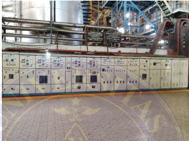
Gambar 3. 68 Panel – Panel Listrik (Main Switch Boarf)
