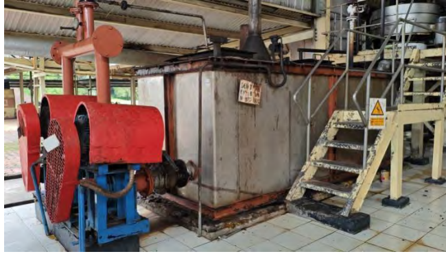
Gambar 3. 25 Diluted Crude Oil Tank
