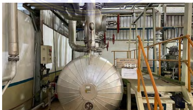
Gambar 3. 65 Back Pressure Vessel
