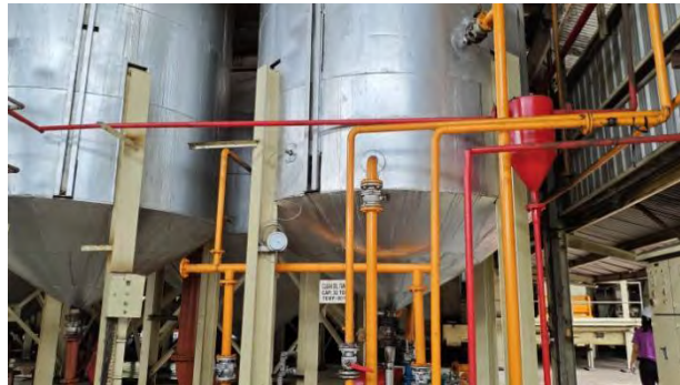
Gambar 3. 29 Clean Oil Tank
