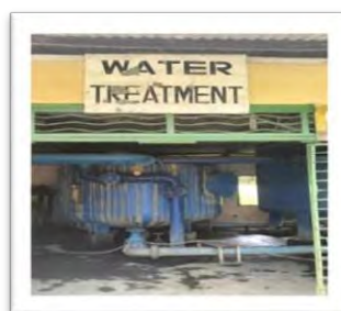
Gambar water treatment
