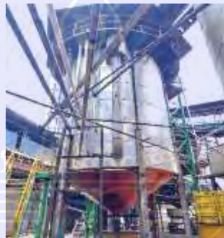
Gambar 3. 20 Vertical Clarifier Tank
