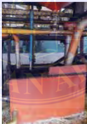
Gambar 3. 30 Sludge Drain Tank
