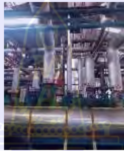
Gambar 3. 41 Back Pressure Vessel
