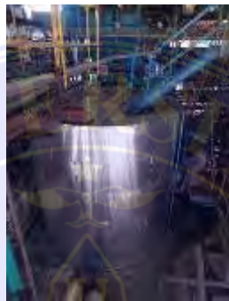
Gambar 3. 50 Feed Water Tank
