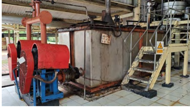
Gambar 3. 21 Diluted Crude Oil Tank
