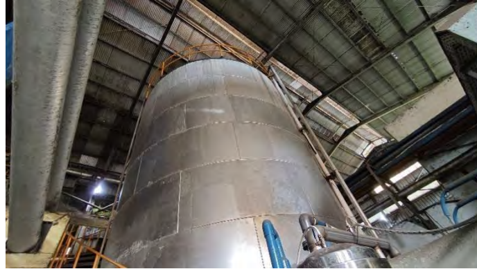
Gambar 3. 58 Feed Water Tank
