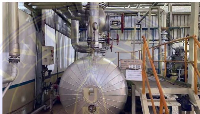
Gambar 3. 61 Back Pressure Vessel
