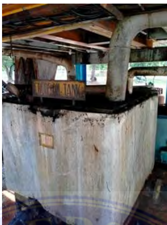
Gambar 3. 17. Crude Oil Tank
