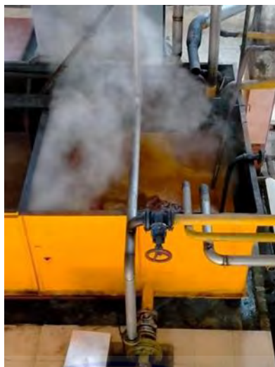
Gambar 3. 24. Oil Collecting Tank
