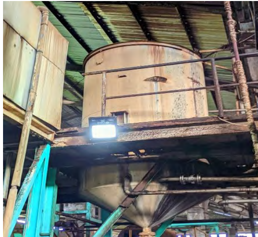
Gambar 3. 23: Hot Water Tank
