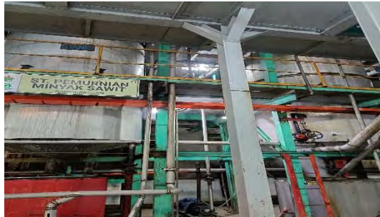
Gambar 3. 16: Clean Oil Tank
