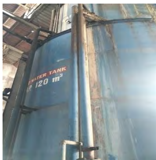
Gambar 3. 43: Feed Water Tank
