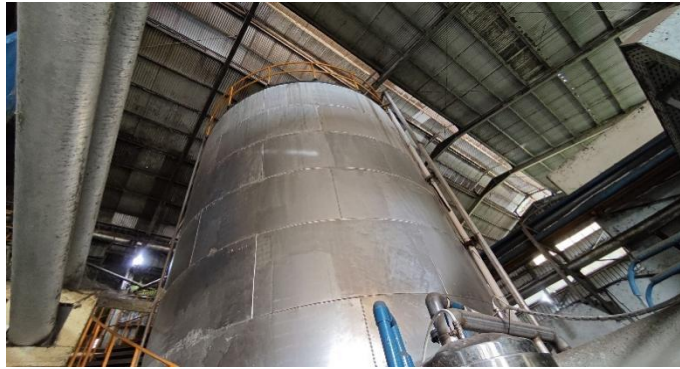
Gambar 3. 62 Feed Water Tank
