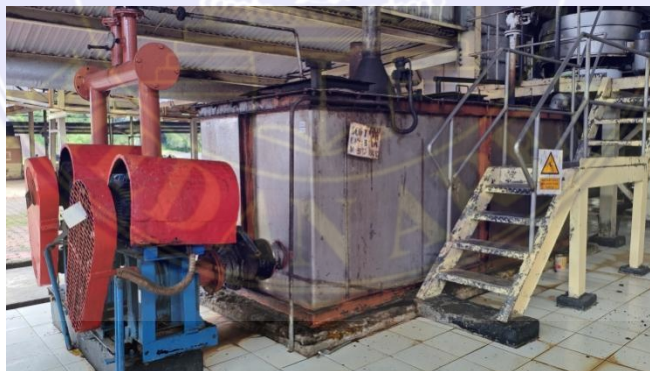
Gambar 3. 25 Diluted Crude Oil Tank
