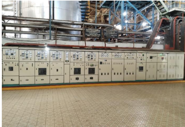
Gambar 3. 68 Panel – Panel Listrik ( Main Switch Boarf )
