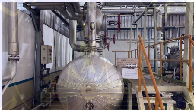
Gambar 3. 65 Back Pressure Vessel
