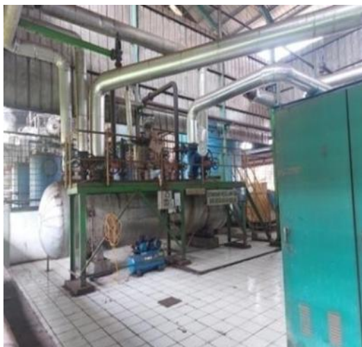
Gambar 3. 76 Back Pressure Vessel
