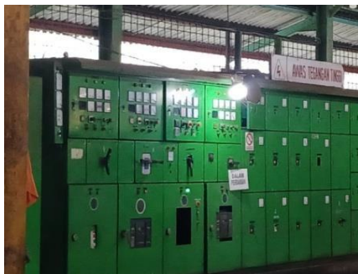
Gambar 3. 78 Main Switch Board
