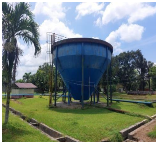
Gambar 3. 80 Water Clarifier Tank
