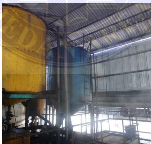
Gambar 3. 50 Hot Water Tank
