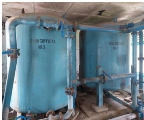
Gambar 3. 84 Sand Filter Tank
