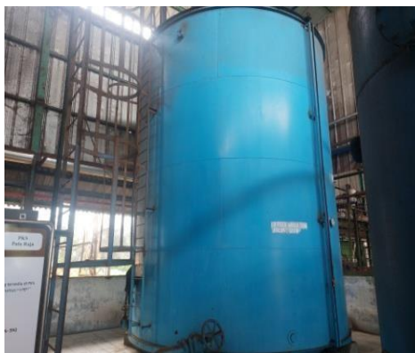
Gambar 3. 90 Boiler feed water tank
