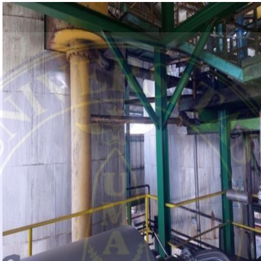
Gambar 3. 34 Continious Settling Tank (CST)
