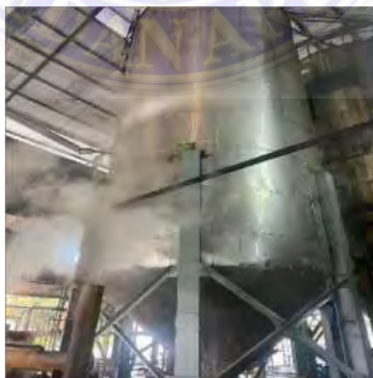
Gambar 3.15 Continous Settling Tank
