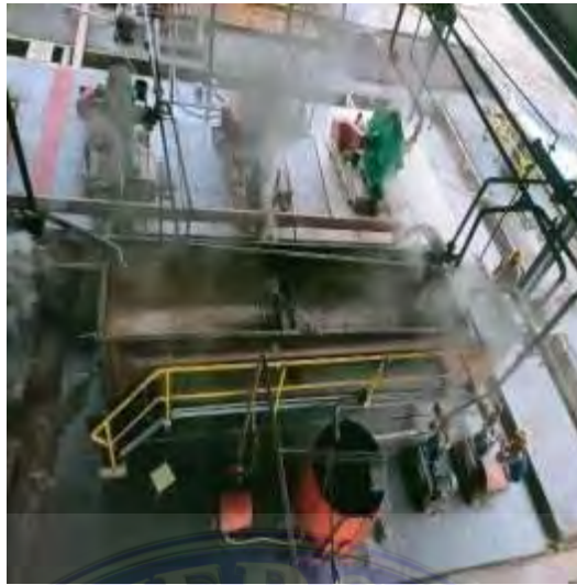
Gambar 3.21 Sludge Drain Tank
