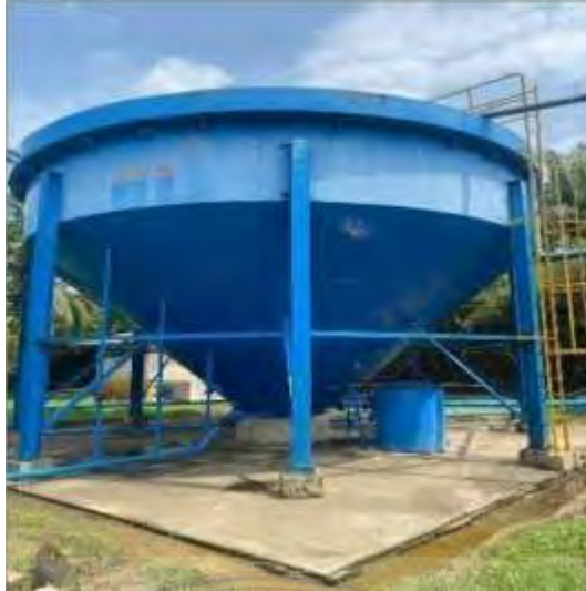
Water Clarifer Tank
