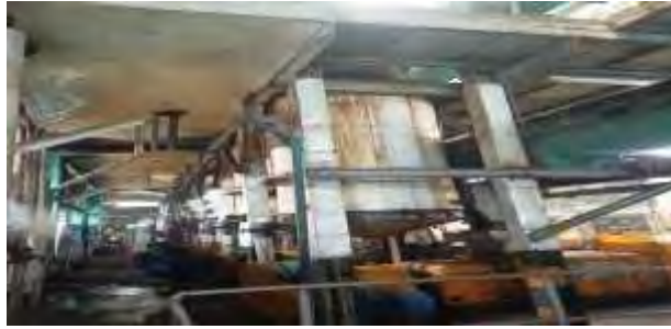
Gambar 3. 26 Crude Oil Tank
