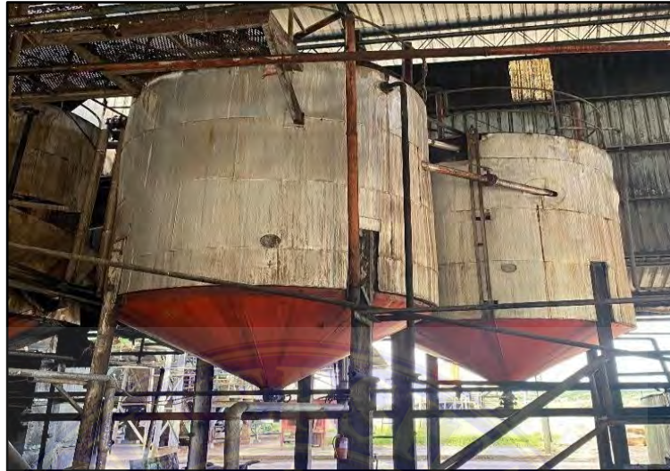
Gambar 3.19 Vertical Clarifier Tank
