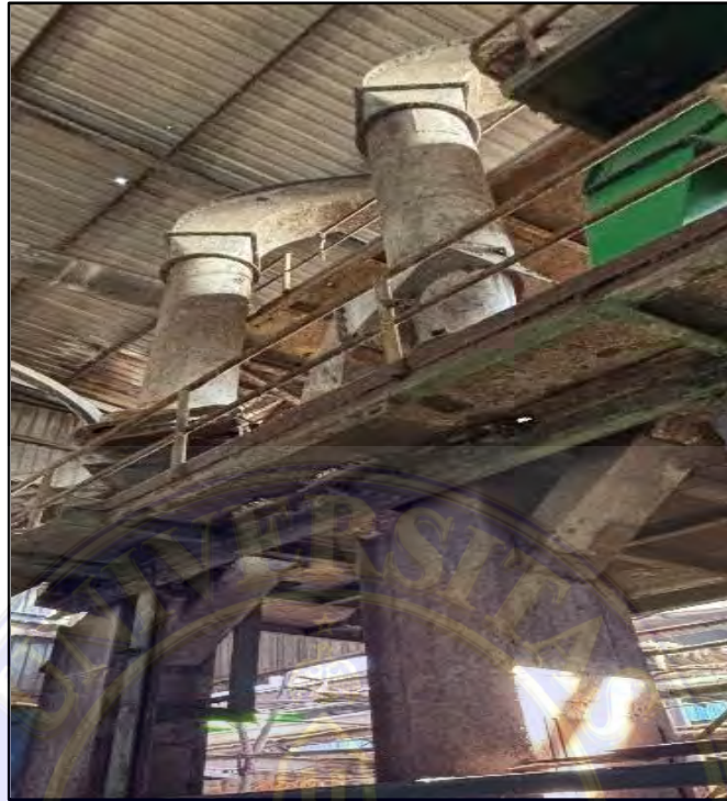
Gambar 3.27 Light Tanera Dust Separation (LTDS)
