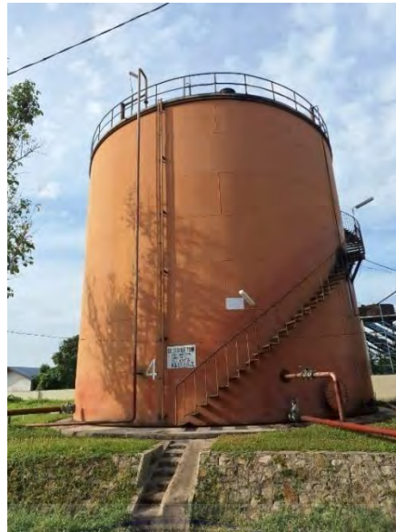
Gambar 3.20 Oil Storage Tank
