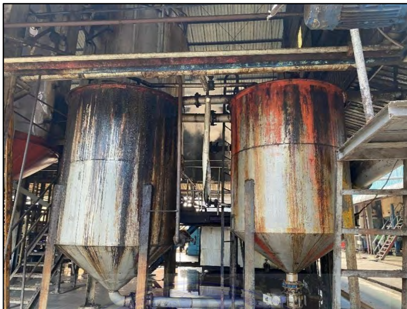
Gambar 3.16 Sand trap tank
