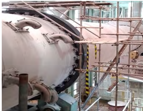
Gambar 3.5 Dryer Rotary Drum (81-M-362)
