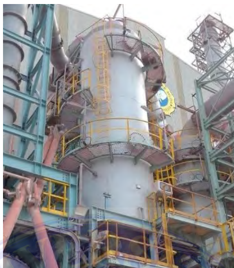
Gambar 3.11 Granulator Prescrubber (81-D-311)
