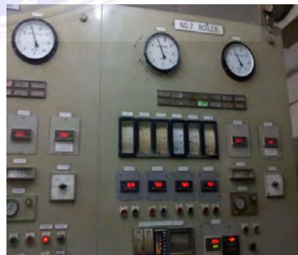
(b) Ruang kontrol Boiler
