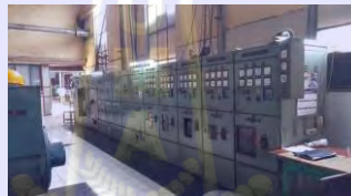
Gambar 3.50 Main Switch Distribution Board ( Panel Kontrol Utama )
