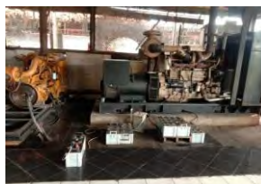
Gambar 3.49 Diesel Angine (Genset)
