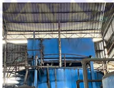
Gambar 3.57 Feed Water Tank
