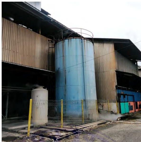
Gambar 3. 64 Feed Water Tank
