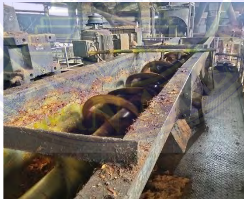
Gambar 3. 24 Top Distributing Conveyor
