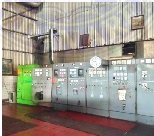
Gambar 3. 57 Main Switch Distribution Board (Panel Kontrol Utama)
