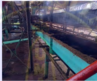
Gambar 3.15 Cake Breaker Conveyer (CBC)
