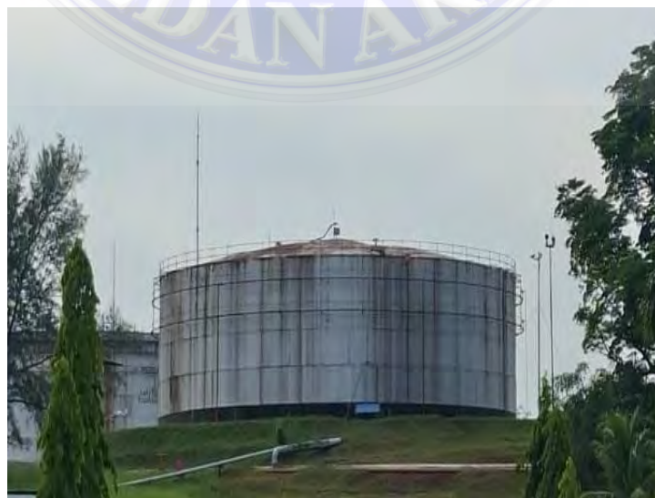
Gambar 3.30 Main Storage Tank (Tangki Timbun Utama)
