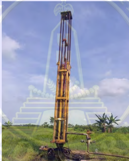
Gambar 3. 6 Hydraulic Pumping unit
