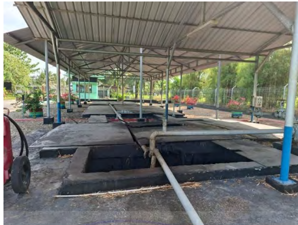
Gambar 3. 35 Cellar Tank (Selobak)
