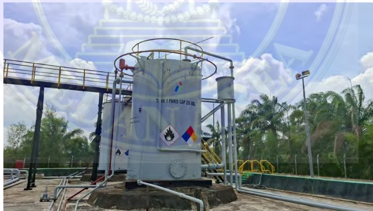
Gambar 3. 33 Tangki Free Water Knock Out (FWKO)
