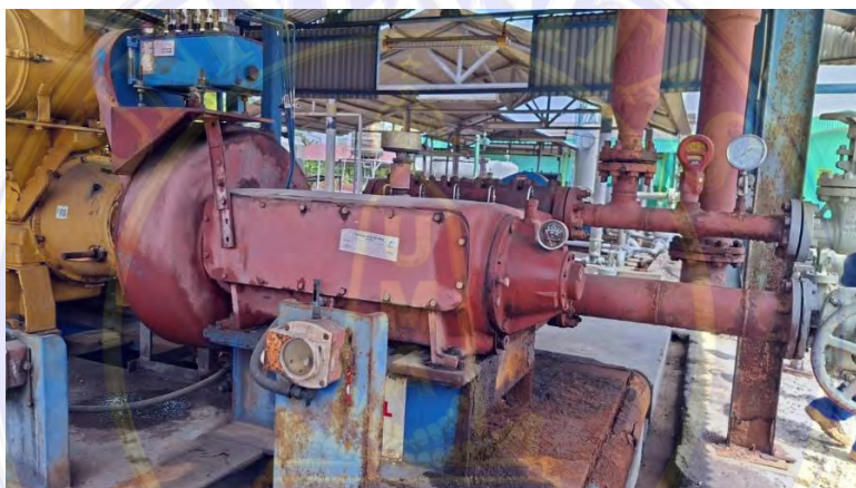
Gambar 3. 34 Pompa Water Injection Plant (WIP)
