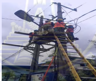
Gambar Perawatan Trafo Distribusi
