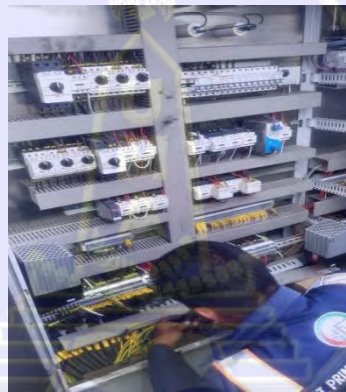
Gambar 3.8. Elektrik Room Rubber Tyred Gantry Craner
