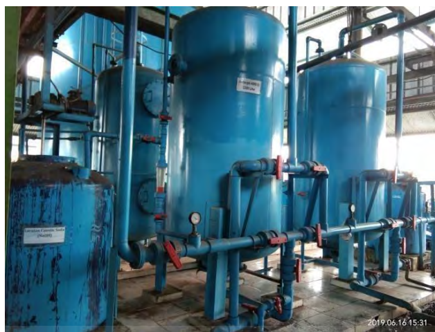
Gambar 3.55. Anion Tank dan Kation Tank
