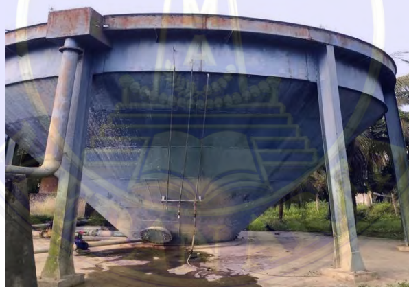
Gambar 3.51. Water Clarifier Tank
