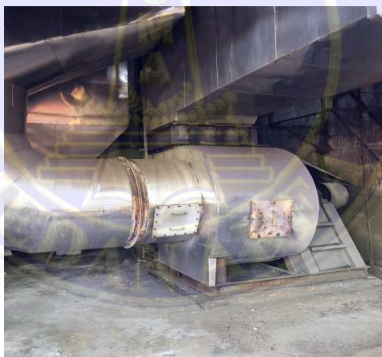
Gambar 3.47. Induced Draft Fan
