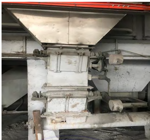
Gambar 3.48. Damper Dust Collector
