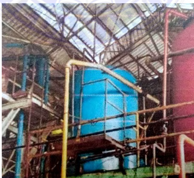
Gambar 3. 30 Hot Water Tank
