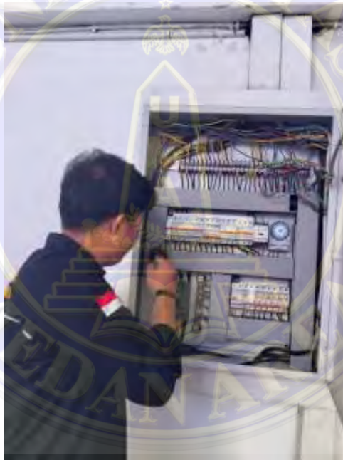
Gambar 2. 3 Panel Utama (Main Distribution Panel/ MDP)
