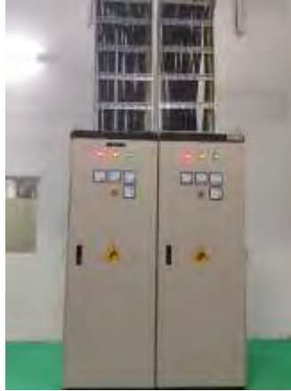
Gambar 2. 1 Panel Utama (Main Distribution Panel/ MDP)
