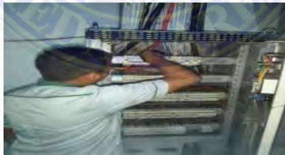
Gambar 2. 2 Panel Cabang (Sub Distribution Panel/ MDP)
