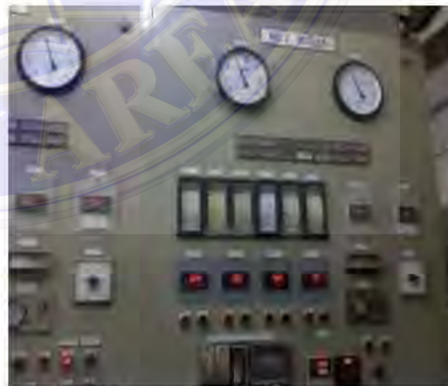
(b) Ruang kontrol Boiler
