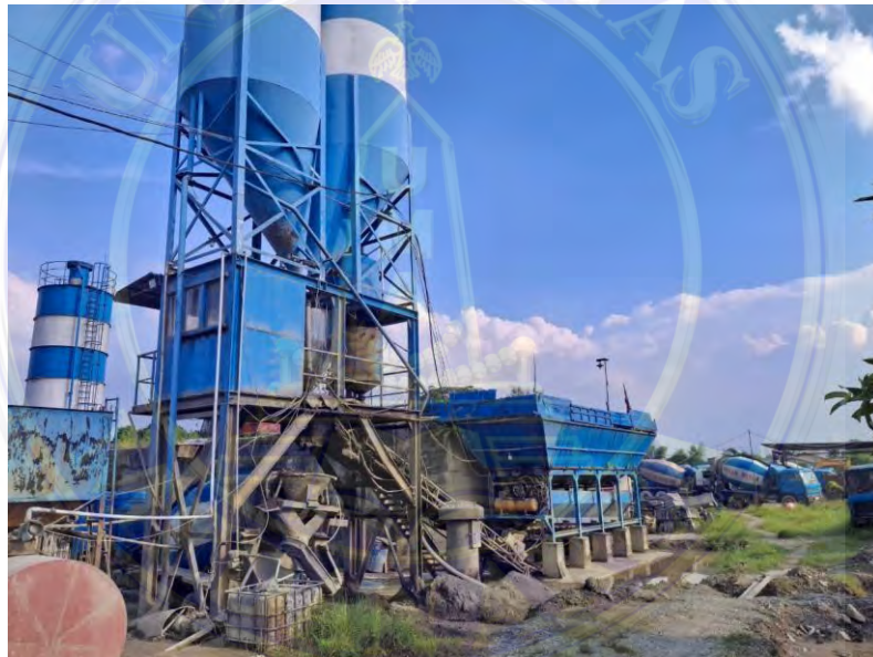
Gambar 3.2. Batching Plant (Dokumentasi,2025)
