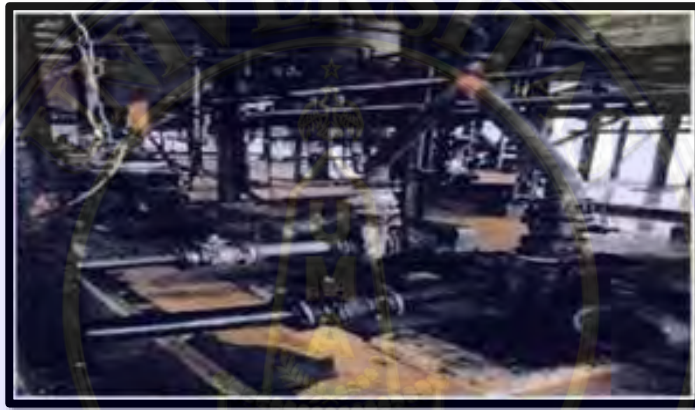
Gambar 3. 19 Oil Transfer Pump
