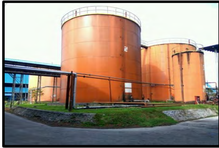
Gambar 3. 20 Oil Storage Tank Gambar
