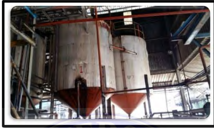
Gambar 3. 14 Sand Trap Tank
