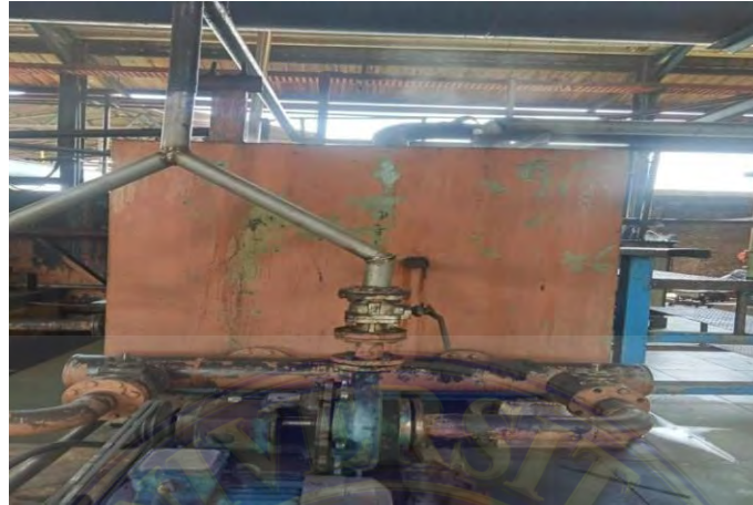
Gambar 3. 16 Light Phase Tank
