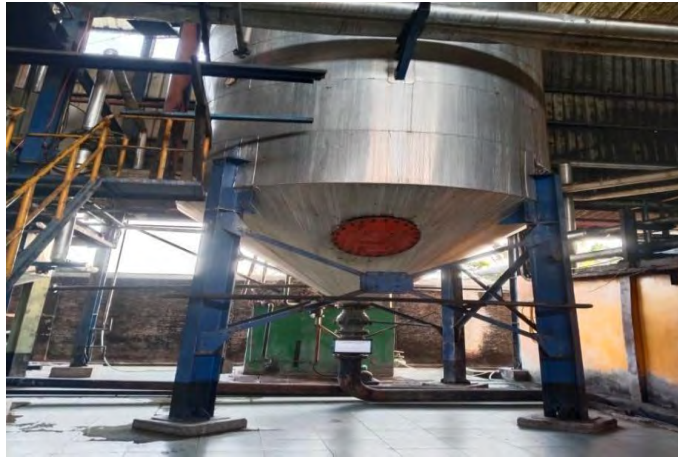
Gambar 3. 12 Continuous Settling Tank
