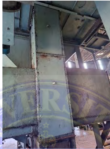
Gambar 3.55 Cracked Mixture Elevator
