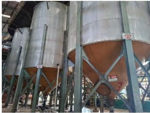
Gambar 3.38 Continuous Settling Tank (CST)
