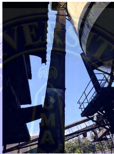
Gambar 3.59 Dry Kernel elevator
