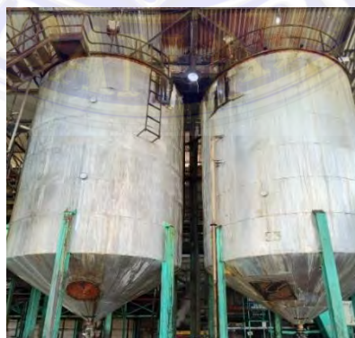
Gambar 3.9 Clarifier Settling Tank (CST)
