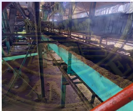
Gambar 3.15 Cake Breaker Conveyer (CBC)
