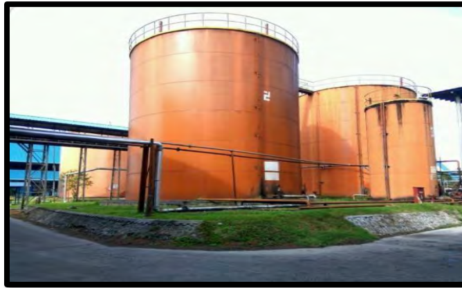
Gambar 3. 20 Oil Storage Tank
