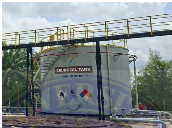
Gambar 3.14 Crude Oil Tank
