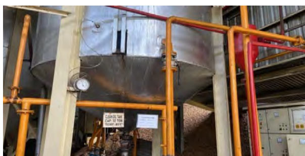
Gambar 3. 25 Clean Oil Tank
