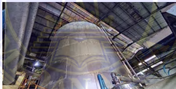
Gambar 3. 58 Feed Water Tank
