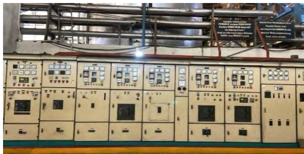
Gambar 3. 64 Panel – Panel Listrik (Main Switch Board)
