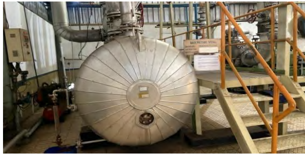
Gambar 3. 61 Back Pressure Vessel
