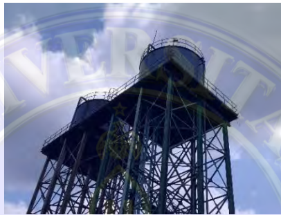
Gambar 3.72 Tower Water Tank
