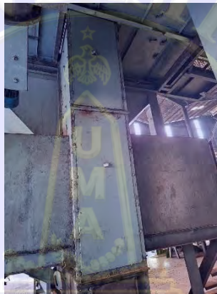
Gambar 3.56 Cracked Mixture Elevator
