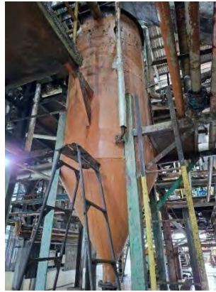
Gambar 3.33 Sand Trap Tank
