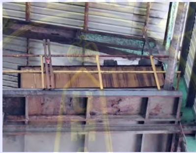
Gambar 3.45 Feeding Separator Tank
