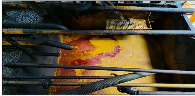
Gambar 3 27 Oil Collecting Tank
