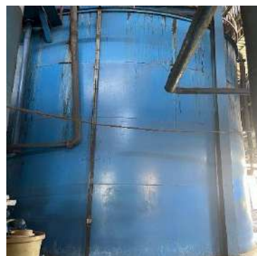
Gambar 4.6 Feed Water Tank
