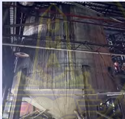
Gambar 3 22 Continuous Settling Tank
