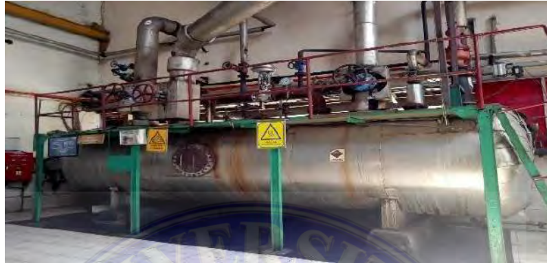
Gambar 4.11 Back Pressure Vessel
