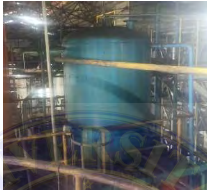
Gambar 3.30 Hot Water Tank
