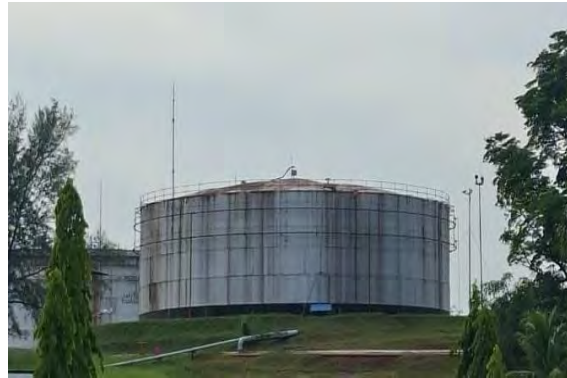
Gambar 3. 30 Main Storage Tank (Tangki Timbun Utama)
