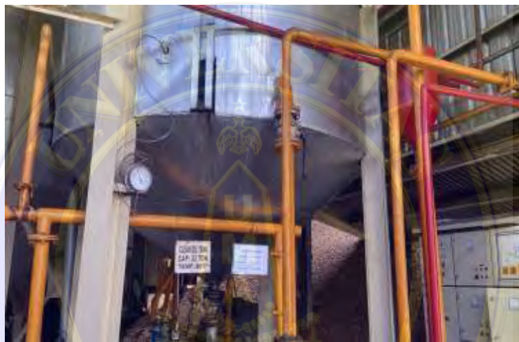
Gambar3.25 Clean Oil Tank
