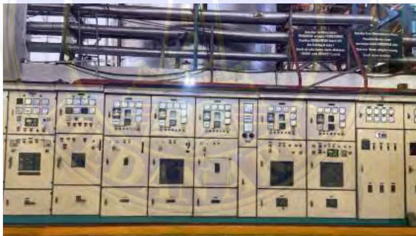
Gambar 3.64 Panel – Panel Listrik ( Main Switch Boarf )
