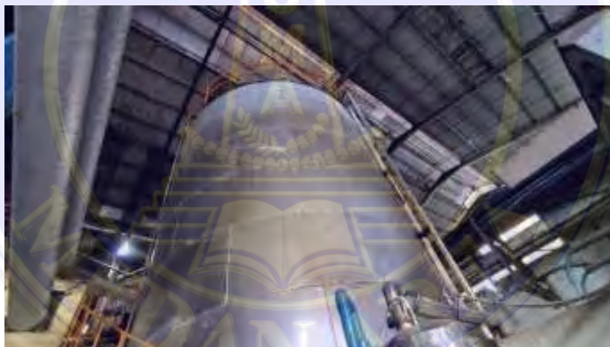
Gambar 3.58 Feed Water Tank
